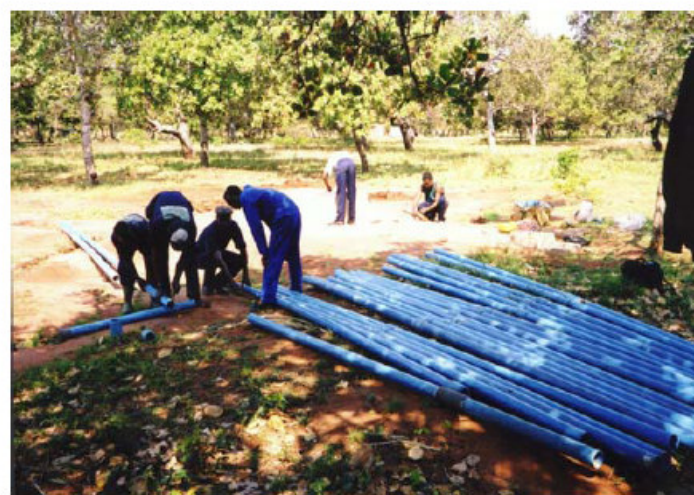
Fig. 6. Installation in a 130 m deep borehole with a water level of 90 m deep; the PVC pipes continue until the bottom of the borehole.
